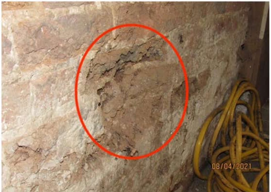
Spalled brickwork on inside surface of workshop north wall
