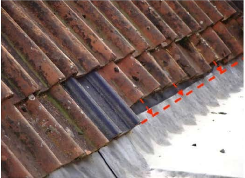
Tiles either broken or incorrectly fixed above central valley gutter
