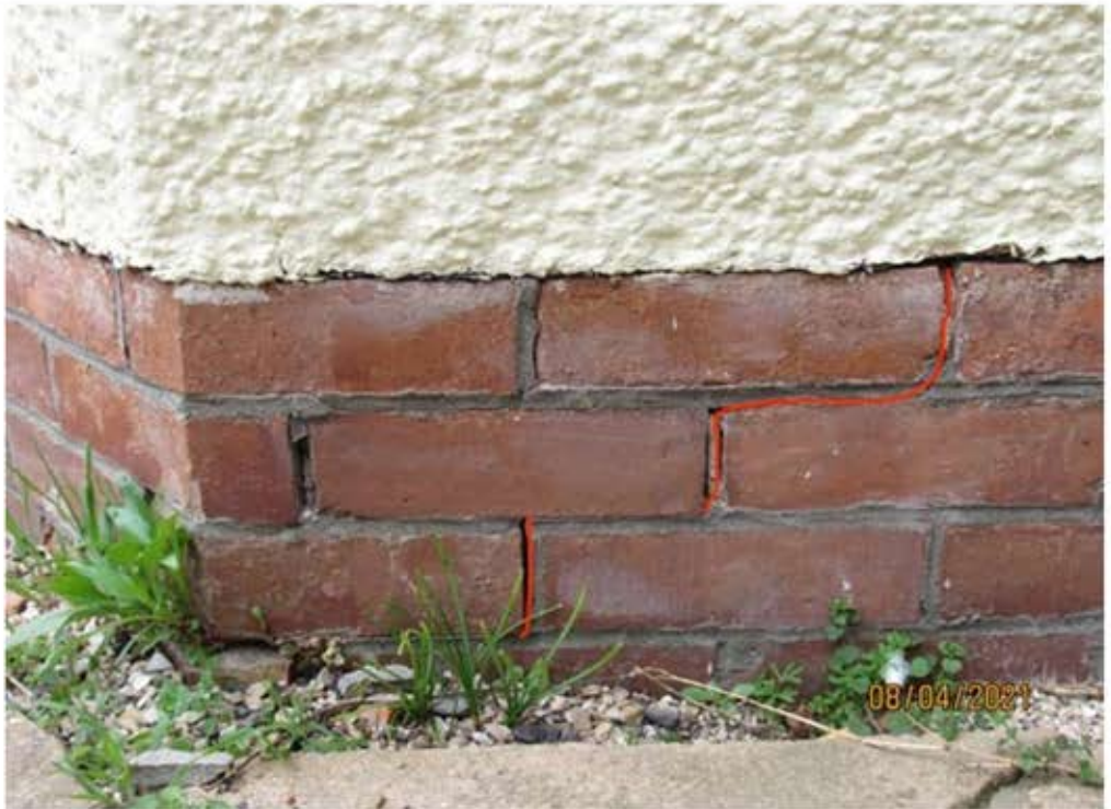
Fine cracking below east bay window
