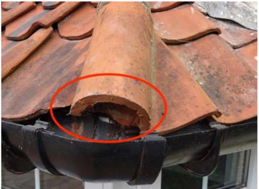
Missing hip iron on both corners of bay roof
