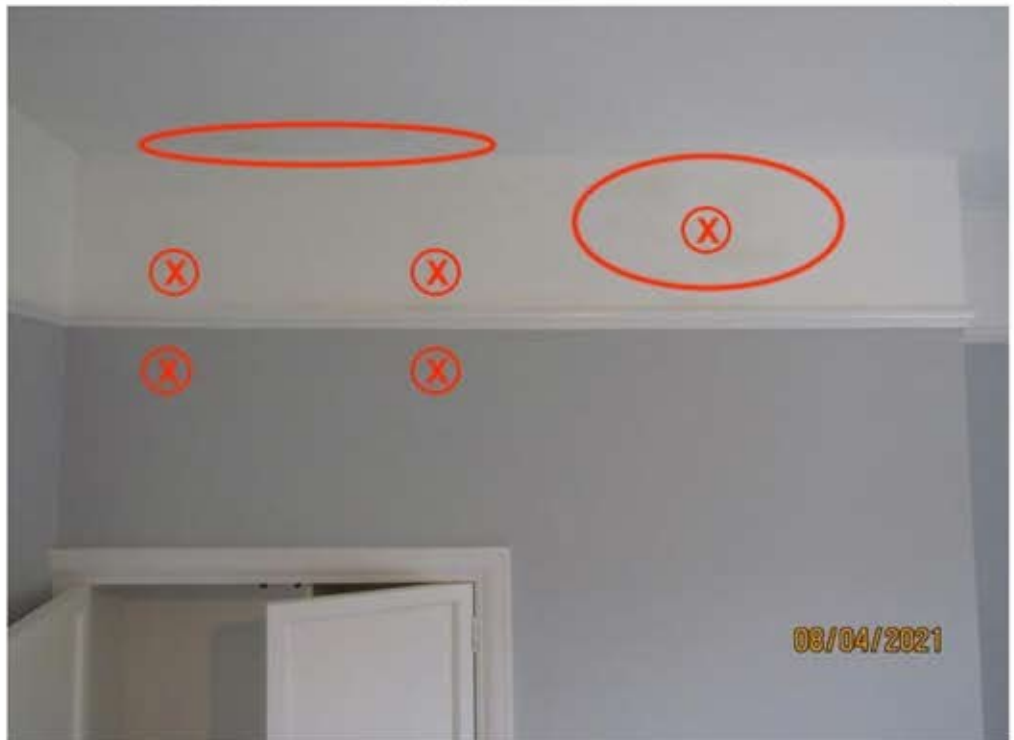
Moisture meter readings in bedroom 3 and areas of water staining
