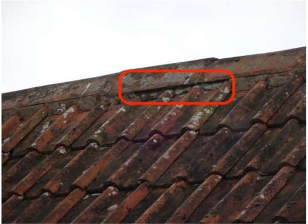
Missing mortar below ridge tiles on east slope
