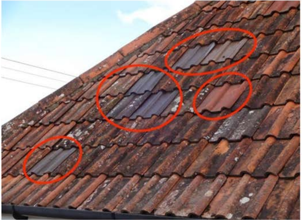
Numerous replacement tiles
