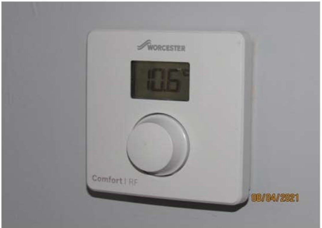
Heating thermostat in utility
