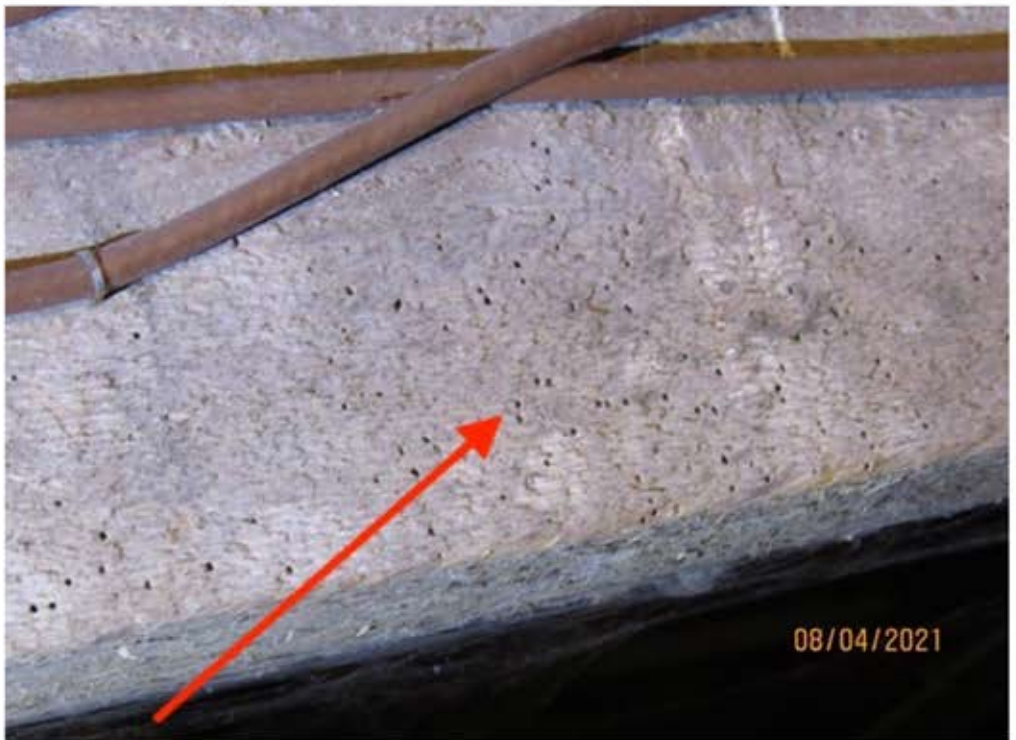
Wood boring insect activity in purlin near access hatch
