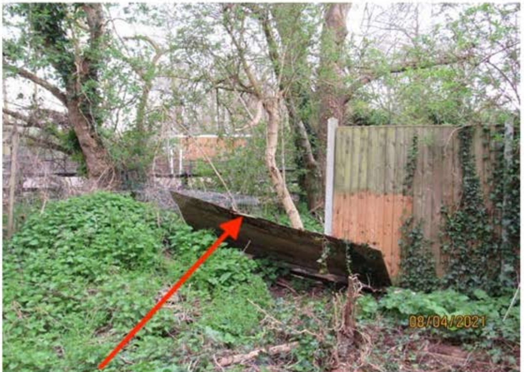
Fallen section of fencing near south-west corner
