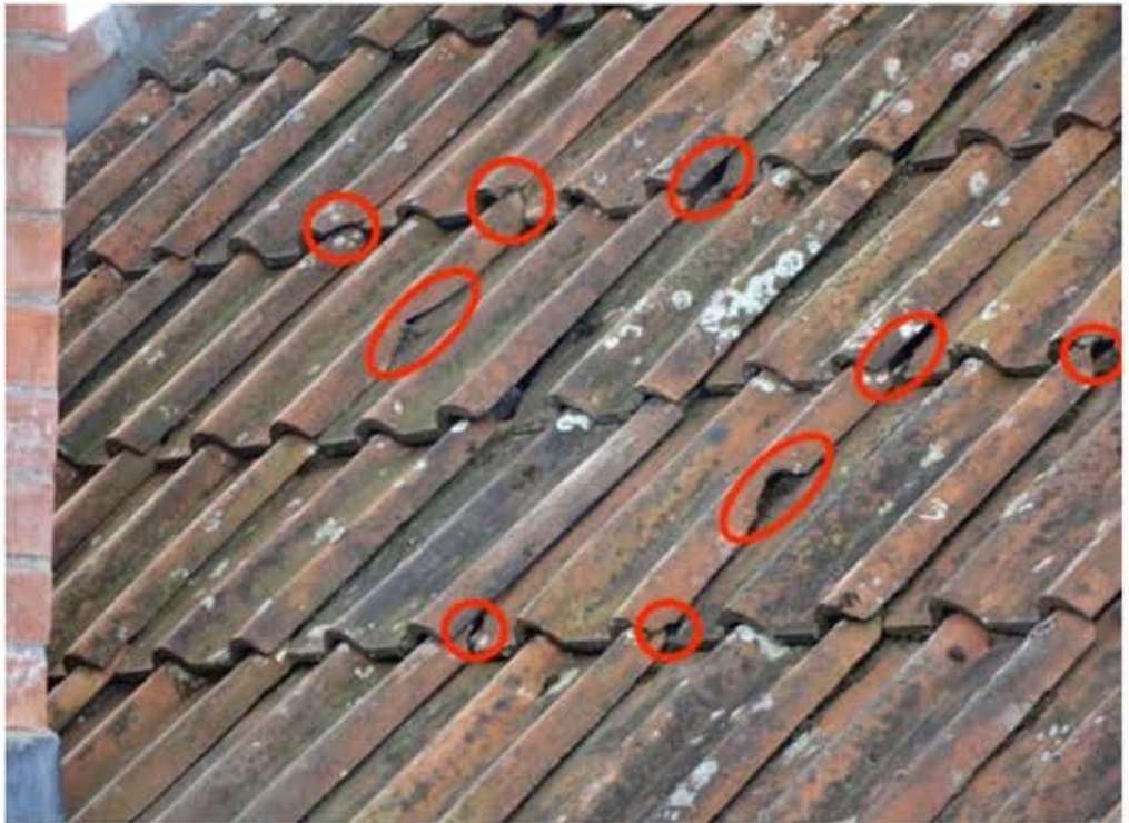
Cracked tiles on east slope
