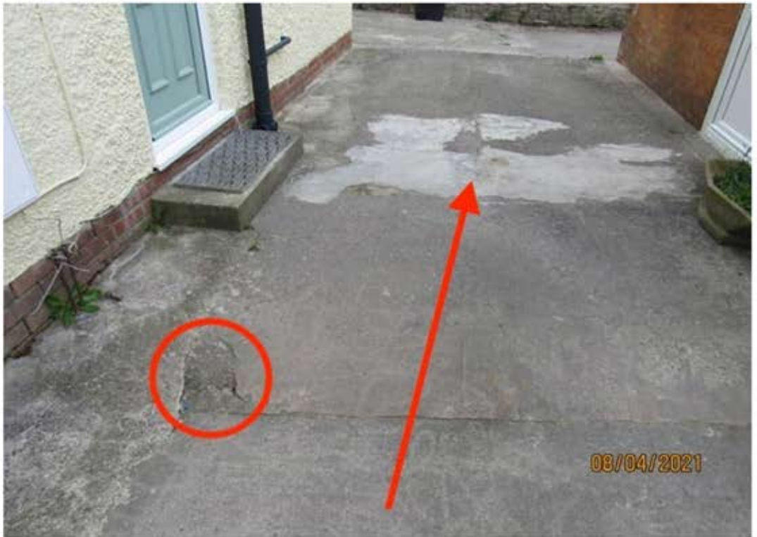
Area of broken surface and patch repairs to driveway
