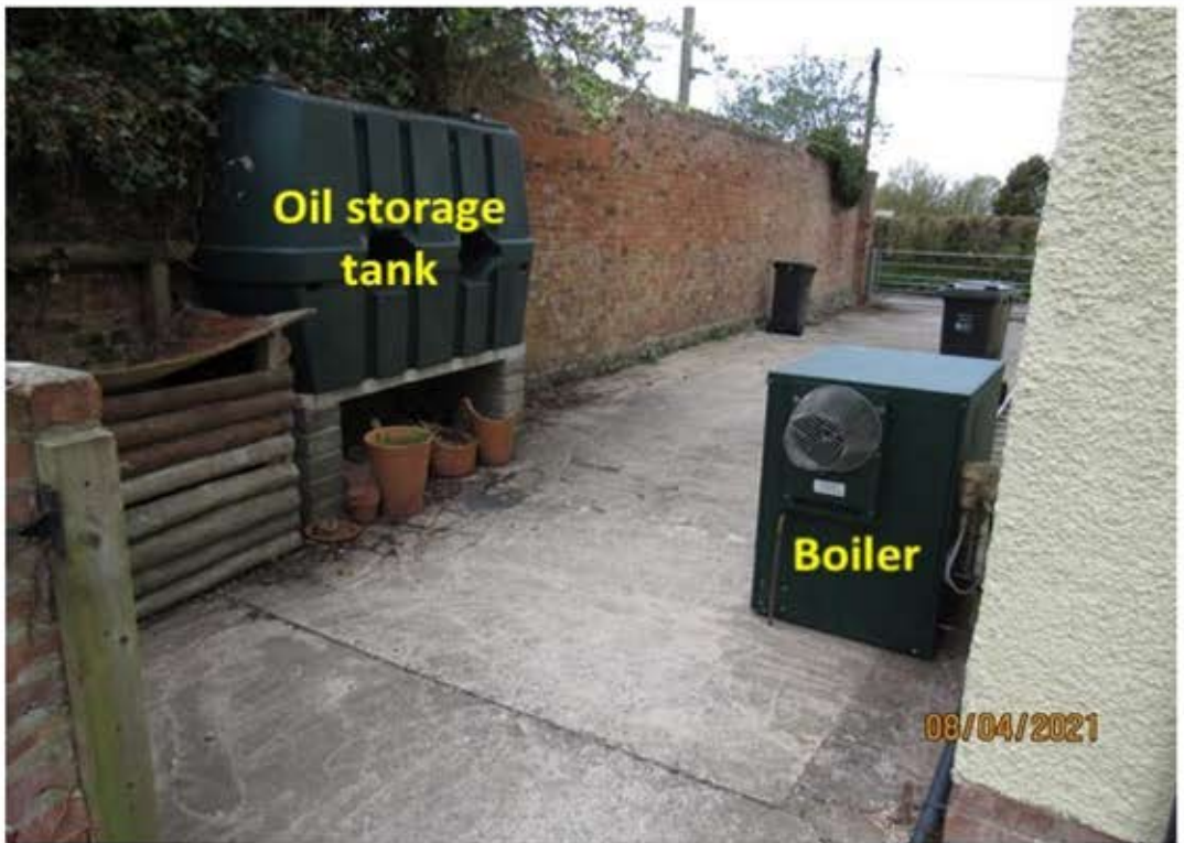
Locations of Oil storage tank and Oil-fired heating system Boiler
