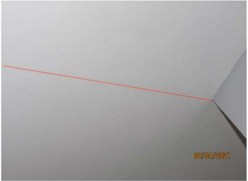
Fine cracking in bedroom 1
