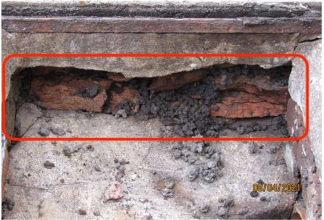
Poor condition of brick chamber wall in IC 1
