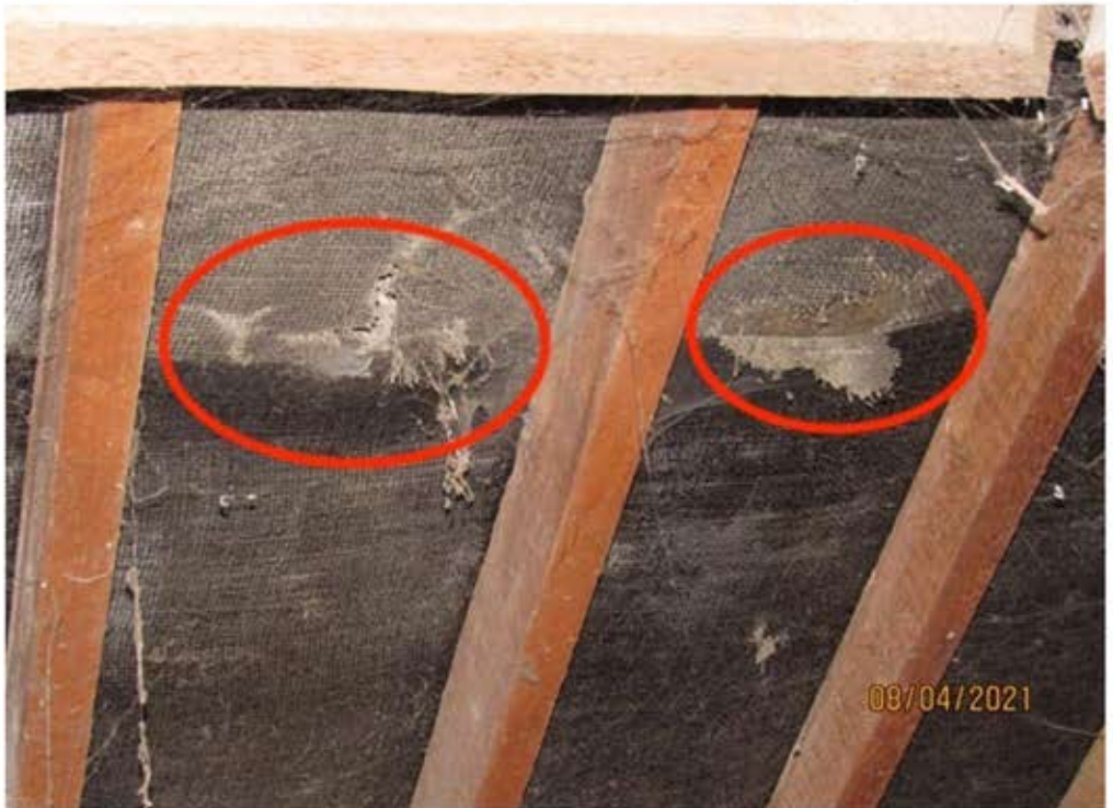
Example of poor condition of bitumen felt underlay
