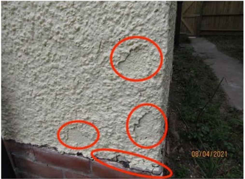
Poor application of render at south-east corner
