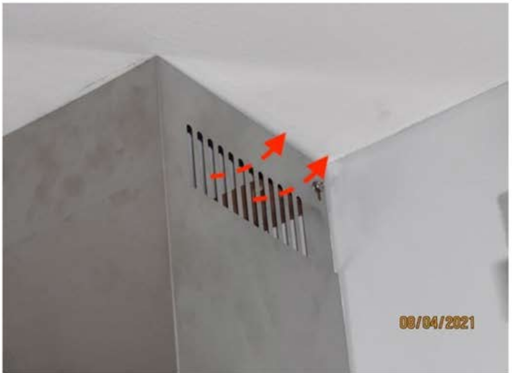
Hood internal ventilation grille
