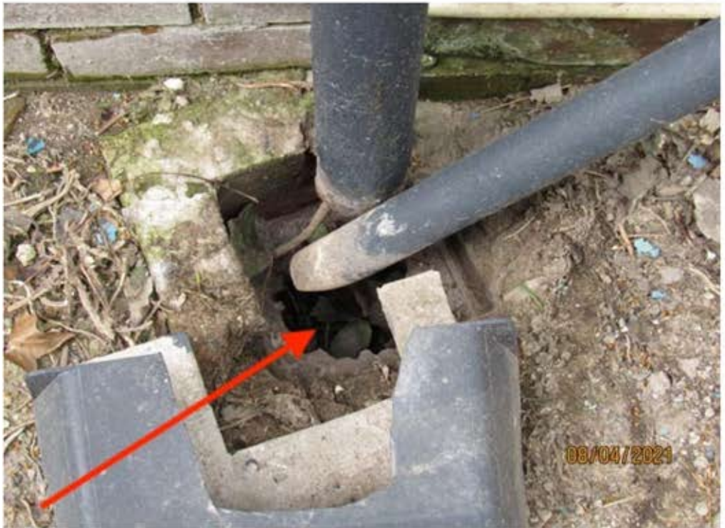
Poor condition of surface gully below east kitchen window
