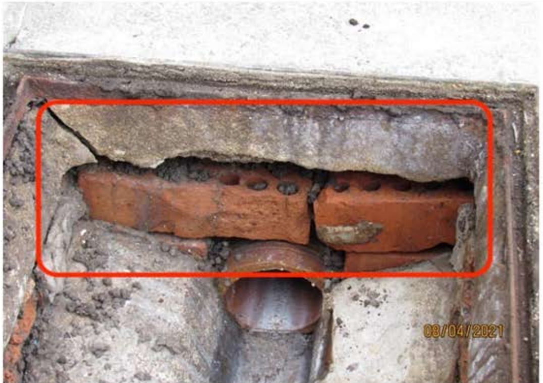
Poor condition of brick chamber wall in IC 1
