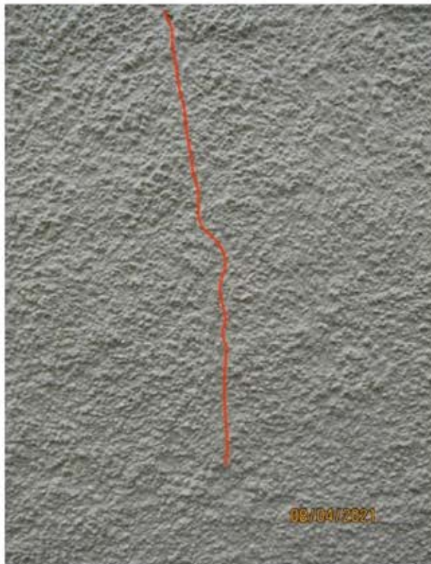
Fine cracking in render on east wall
