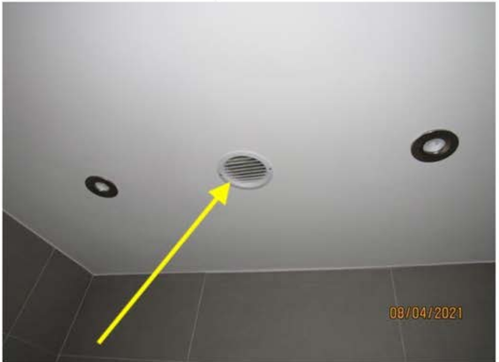
Extractor fan vent in ensuite ceiling
