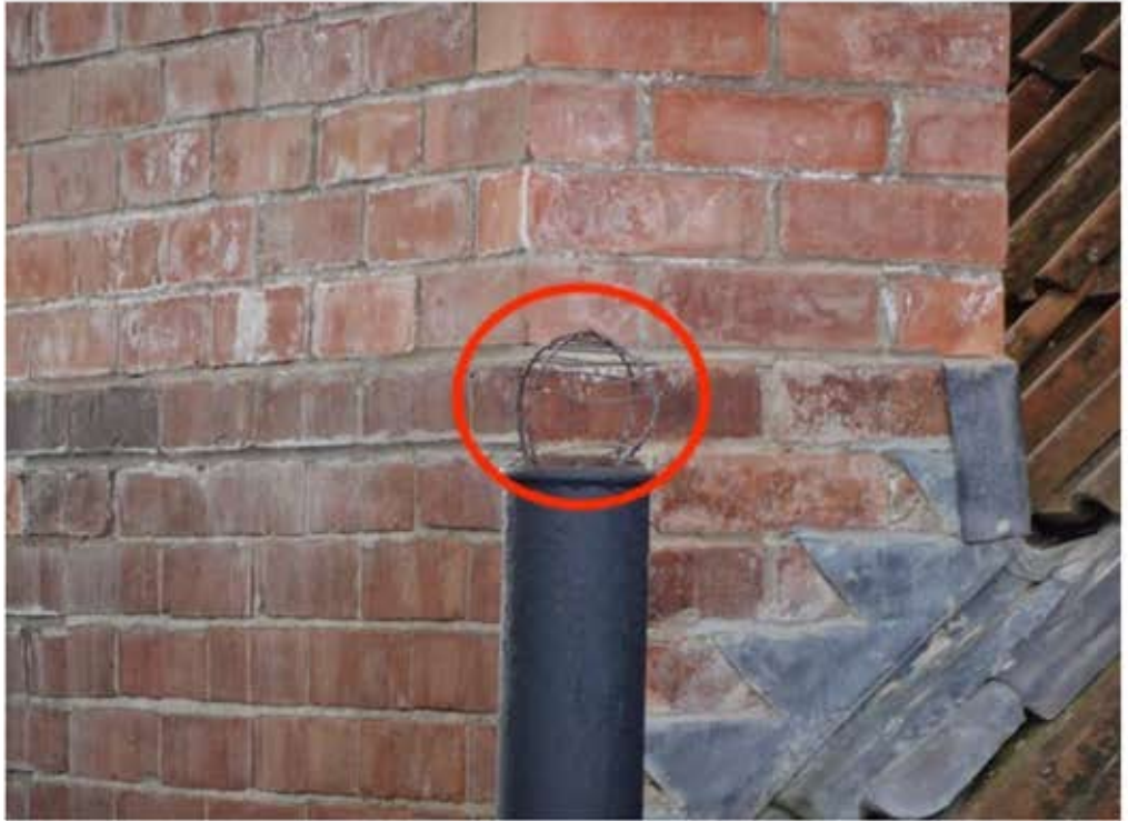
Old worn wire bird guard in east SPV
