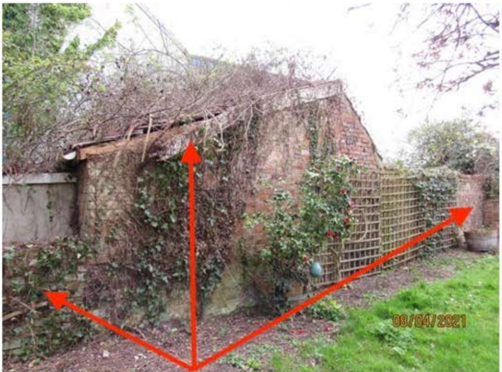
Poor condition of old brick walls and east elevation of neighbour's building
