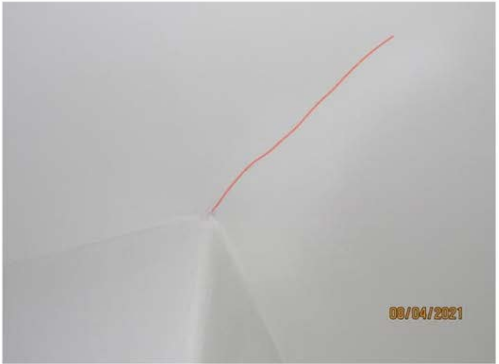
Fine cracking in dining room
