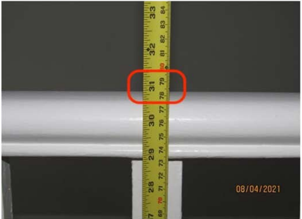
Height of handrail on landing bannister is too low
