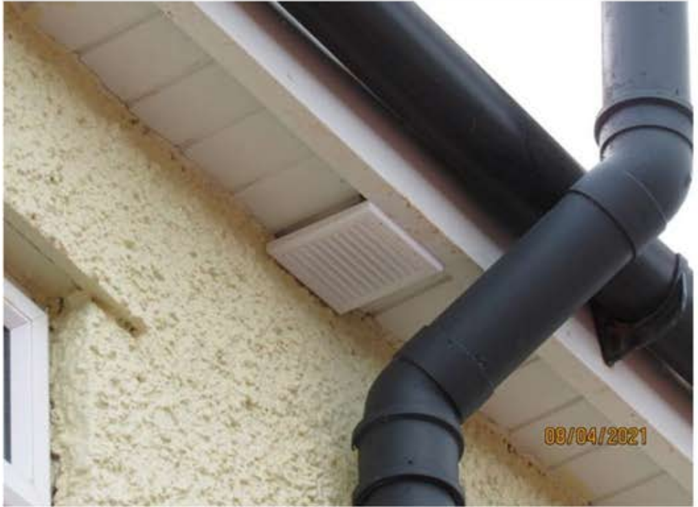
External ventilation grille from ensuite extractor fan
