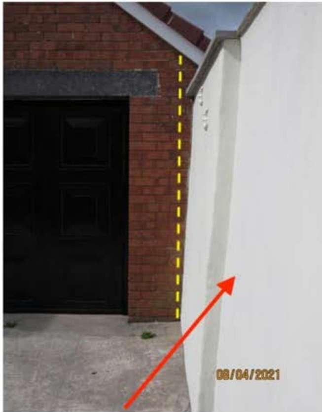
The rendered north boundary wall is leaning towards the road.
