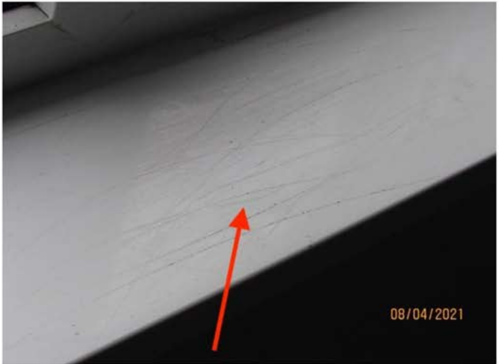
Scratches in window sill
