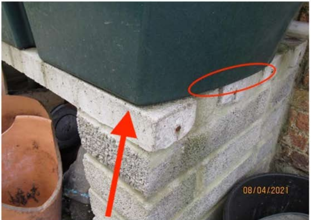
Oil tank support base is too small for size of tank
