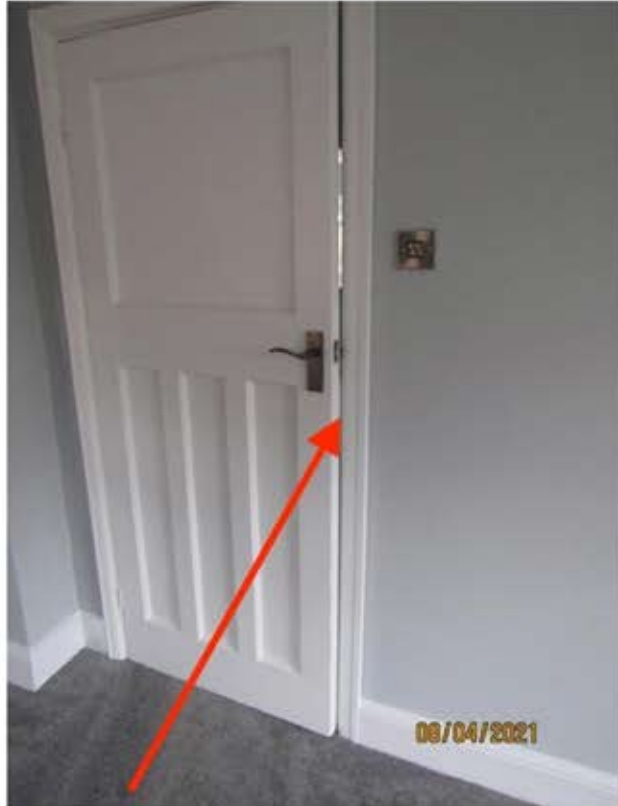
Doors for bedrooms 2 and 3 do not close correctly
