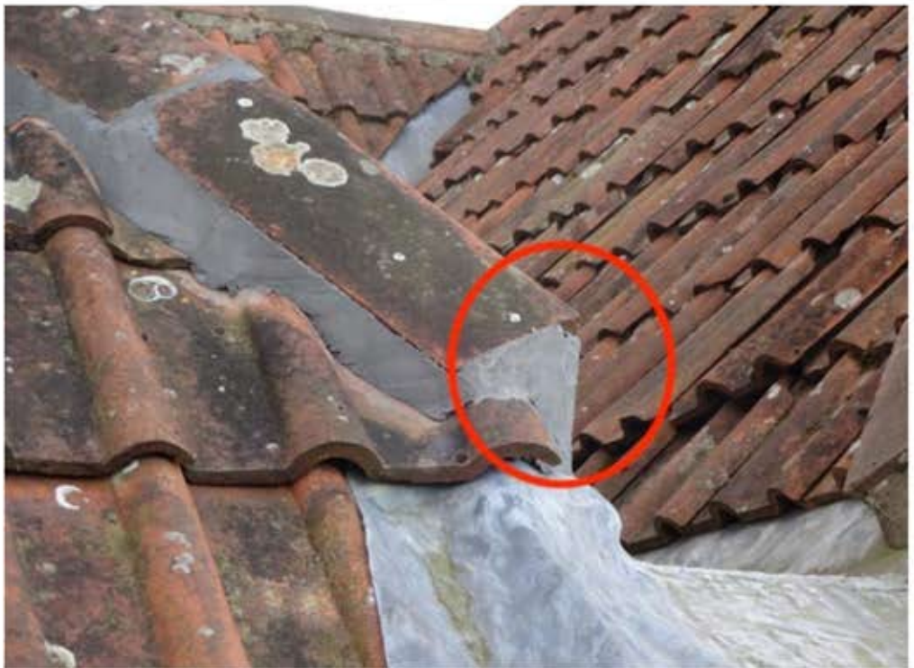
Missing hip iron to secure ridge end tile
