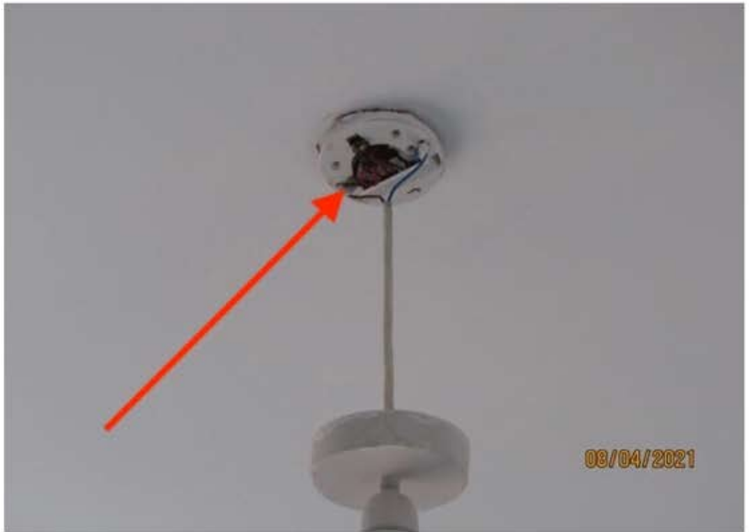
Exposed wiring in bedroom 4 ceiling pendant fitting
