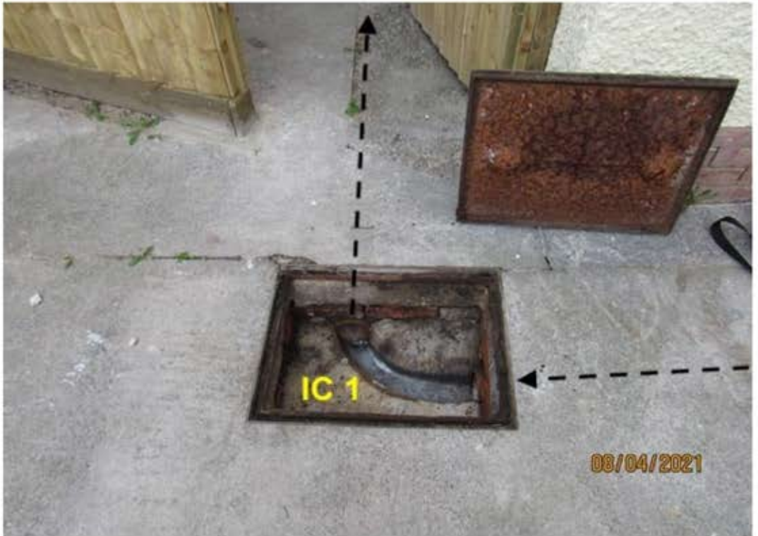
Drainage inspection chamber near north-east corner (IC 1) and estimated position of pipework
