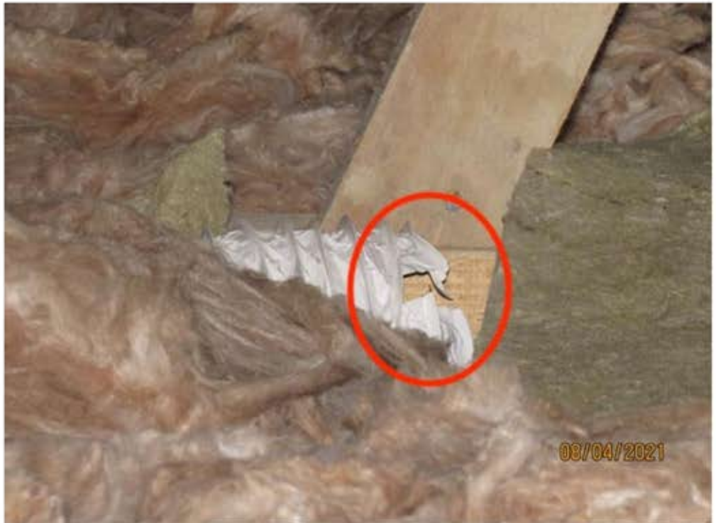
Part of flexible ventilation ducting from ensuite extractor fan to external vent grille in north soffit board
