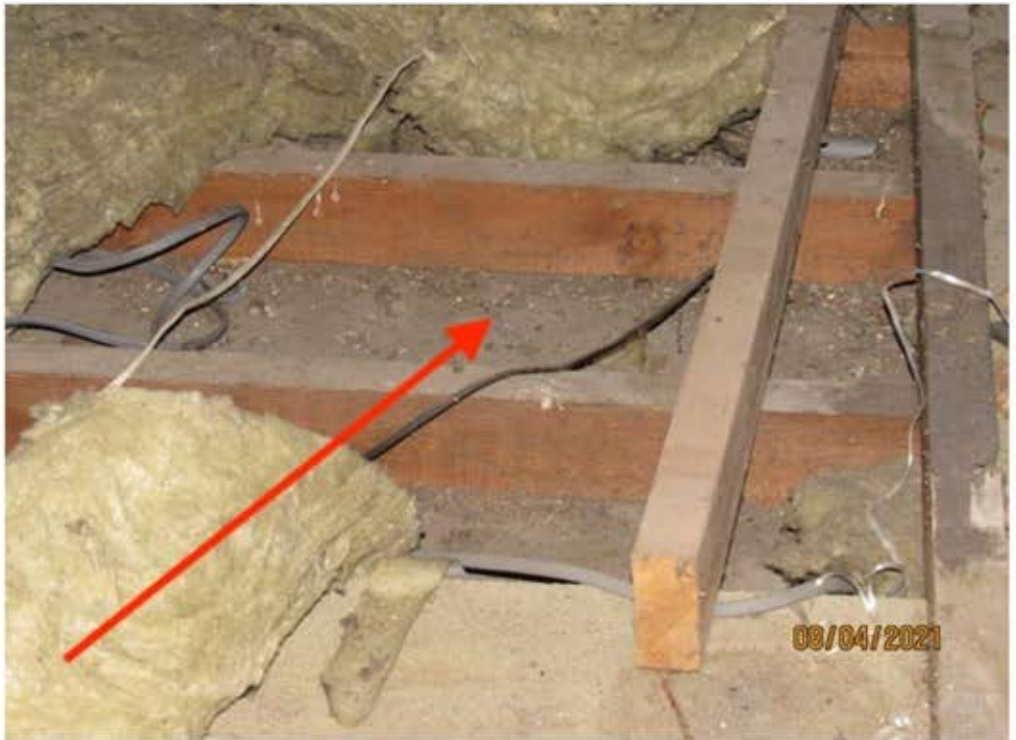
Lack of insulation in some areas
