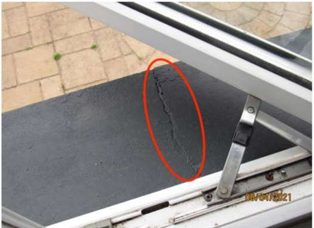
Cracking in bedroom 3 window sill
