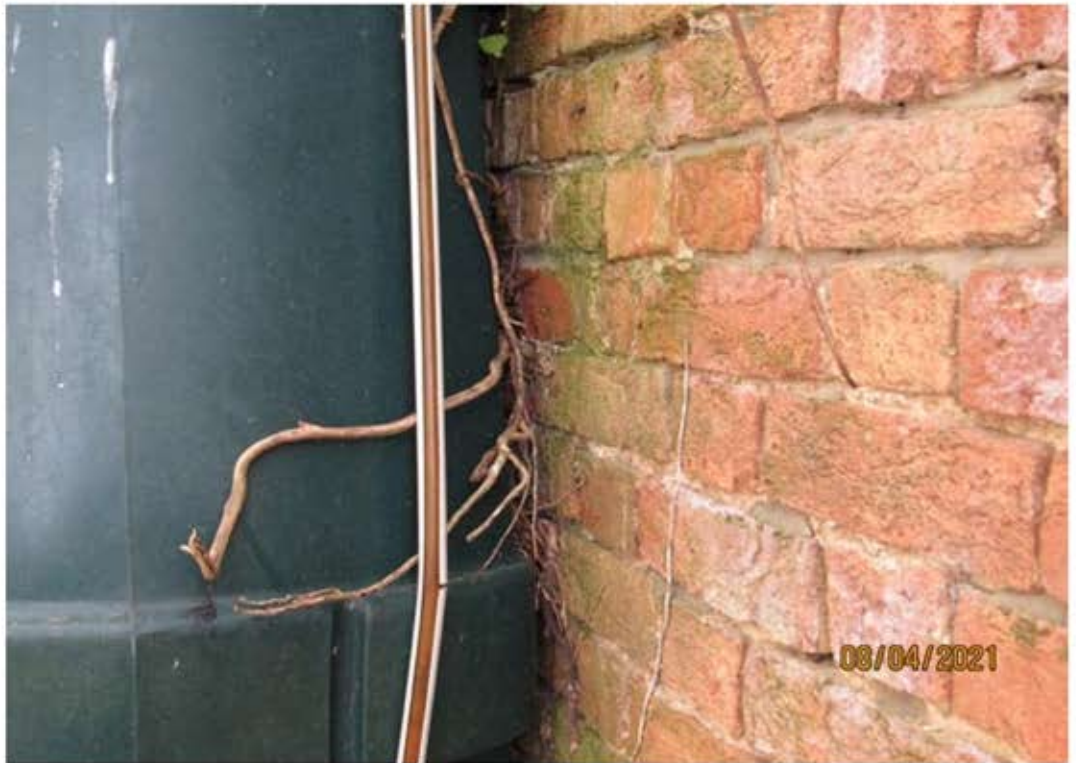
Oil storage tank touching west boundary wall
