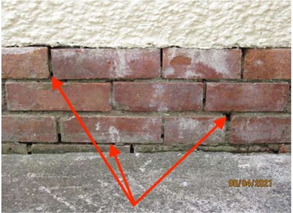
Missing mortar in various location of brick base
