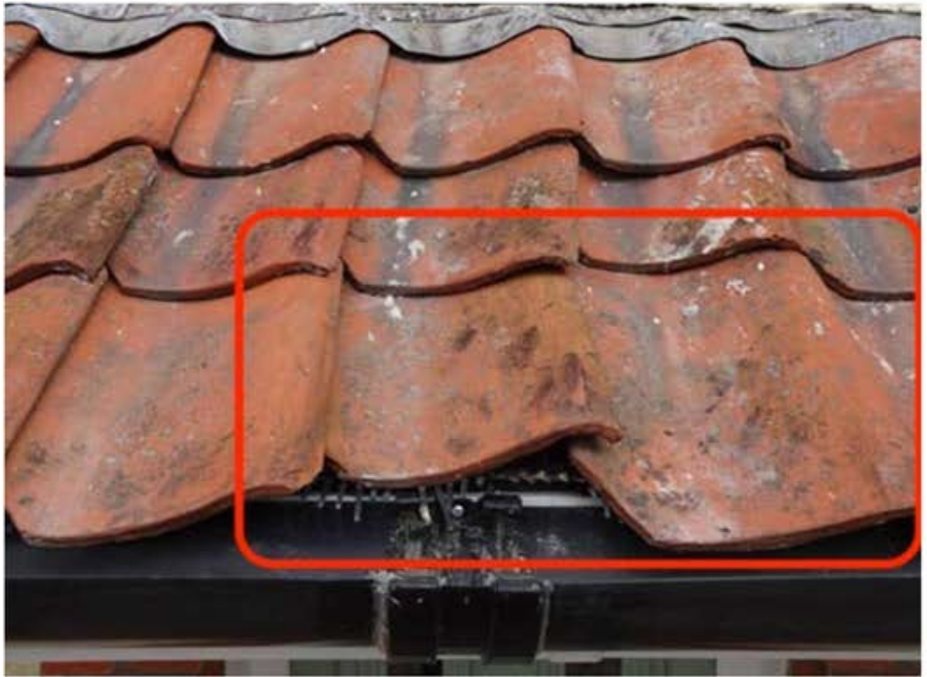
Poor fixing of bay roof tiles
