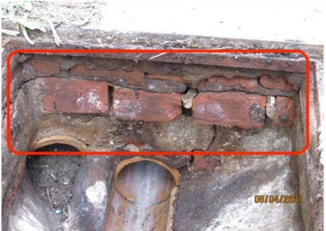
Poor condition of brick chamber wall in IC 2
