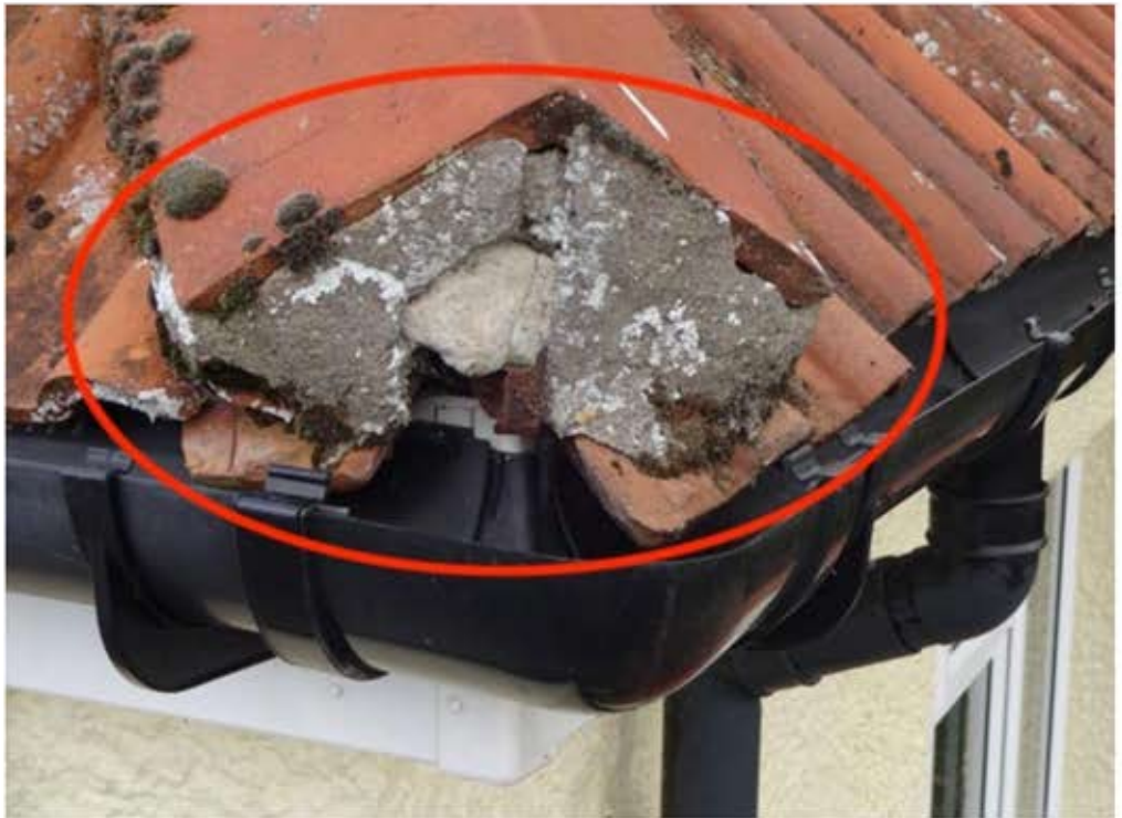
Poor workmanship at south-west corner
