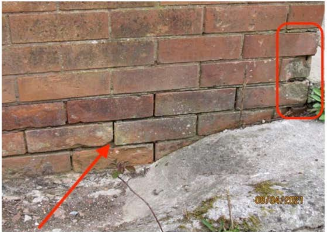
Missing mortar near south-west corner of workshop
