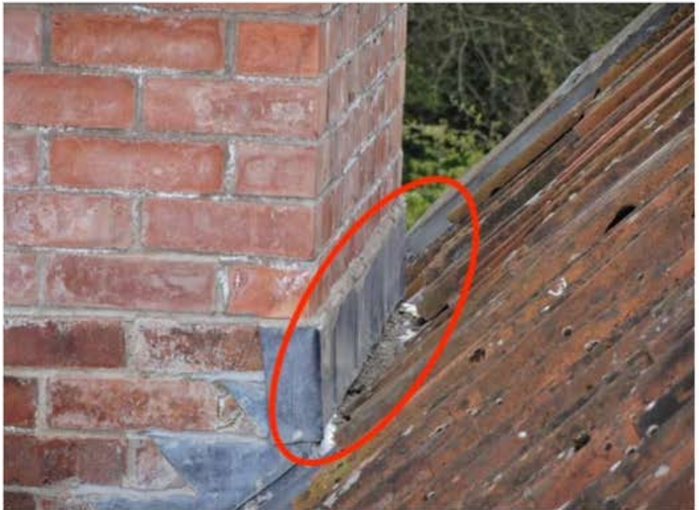
Vulnerable rear gutter on chimney stacks
