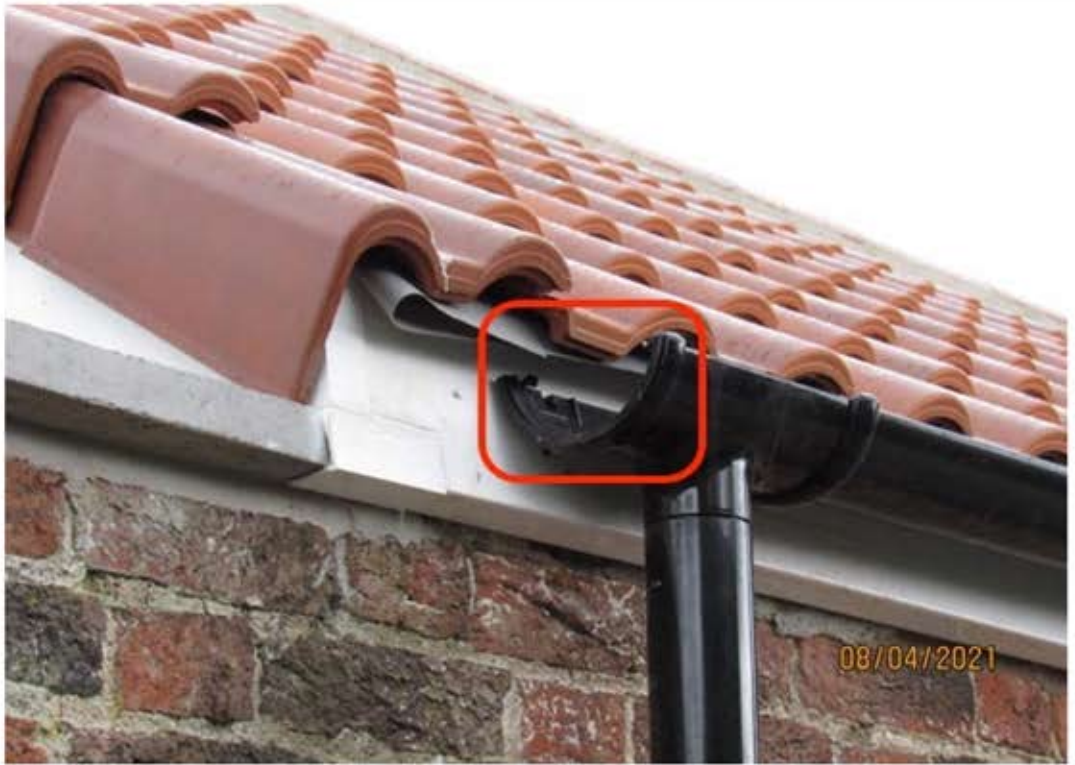
Missing gutter end cap on north-east corner of garage
