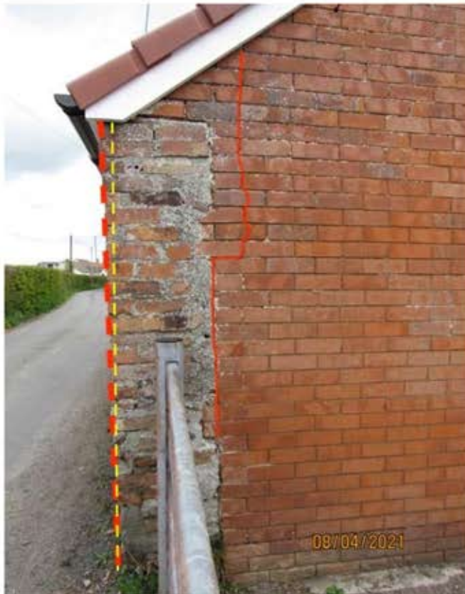
Cracking near north-west corner of workshop and north wall out of plumb
