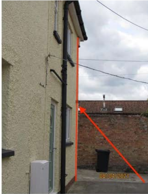
North-west wall bowing slightly
