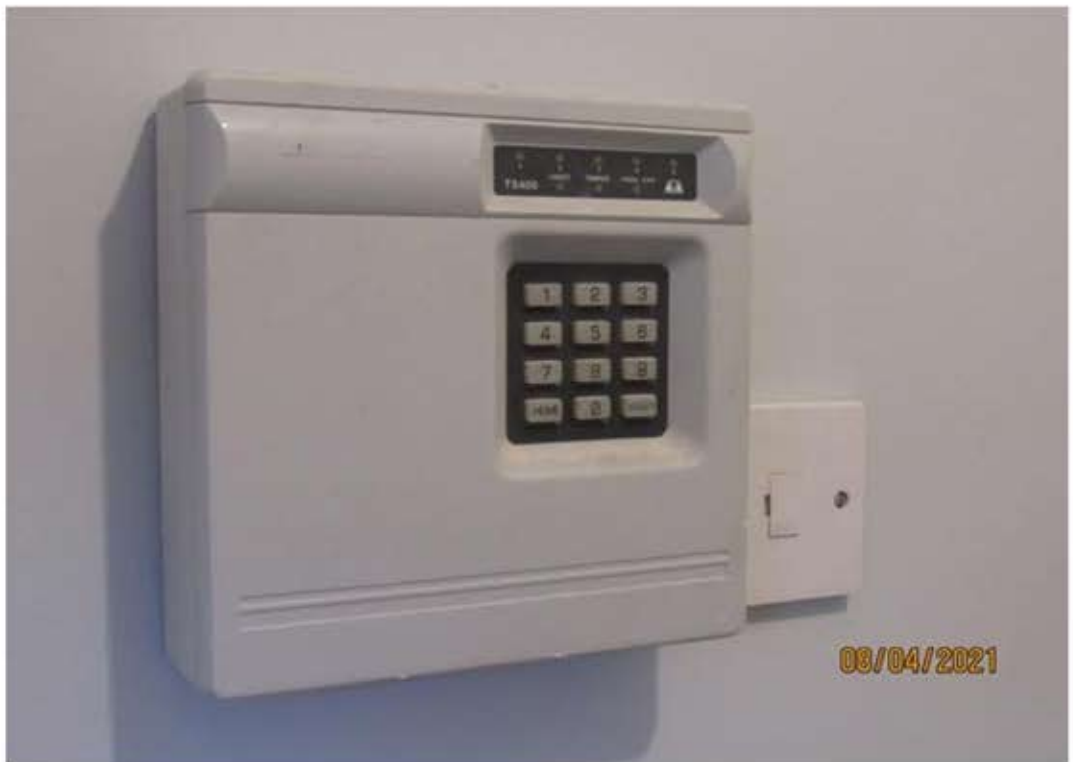
Intruder alarm in cloakroom
