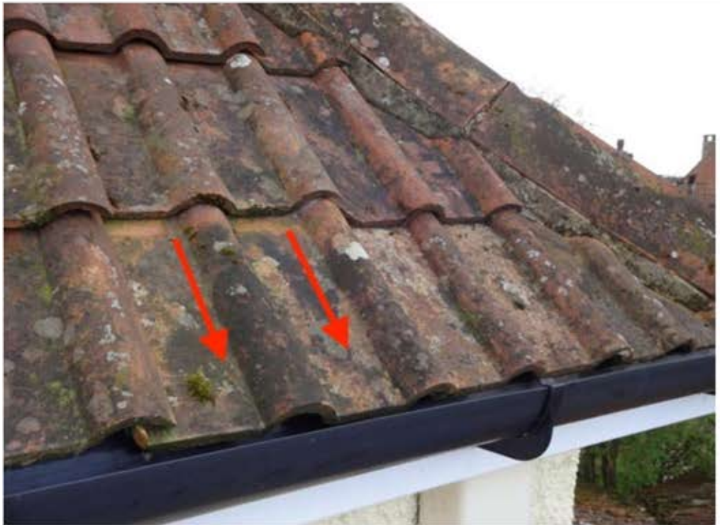
Slipped tiles above gutter
