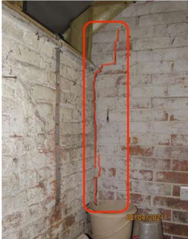
Cracking in partition wall between workshop and garage
