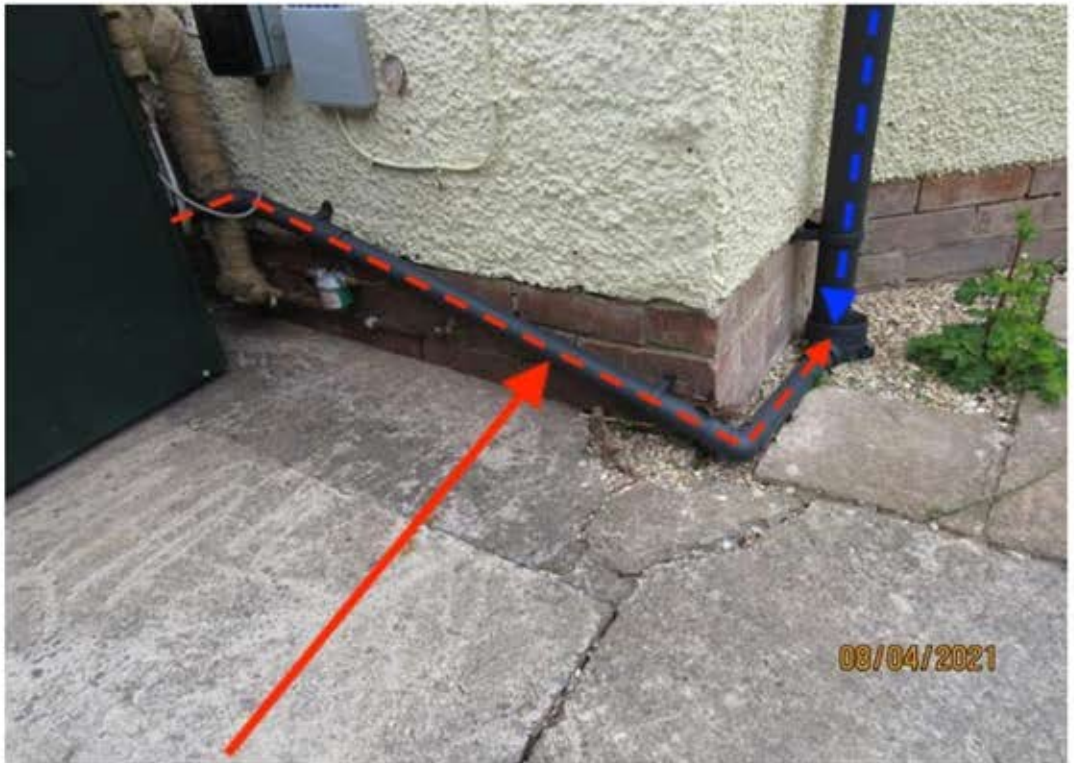
Condensate pipe sharing rainwater gully at south-west corner
