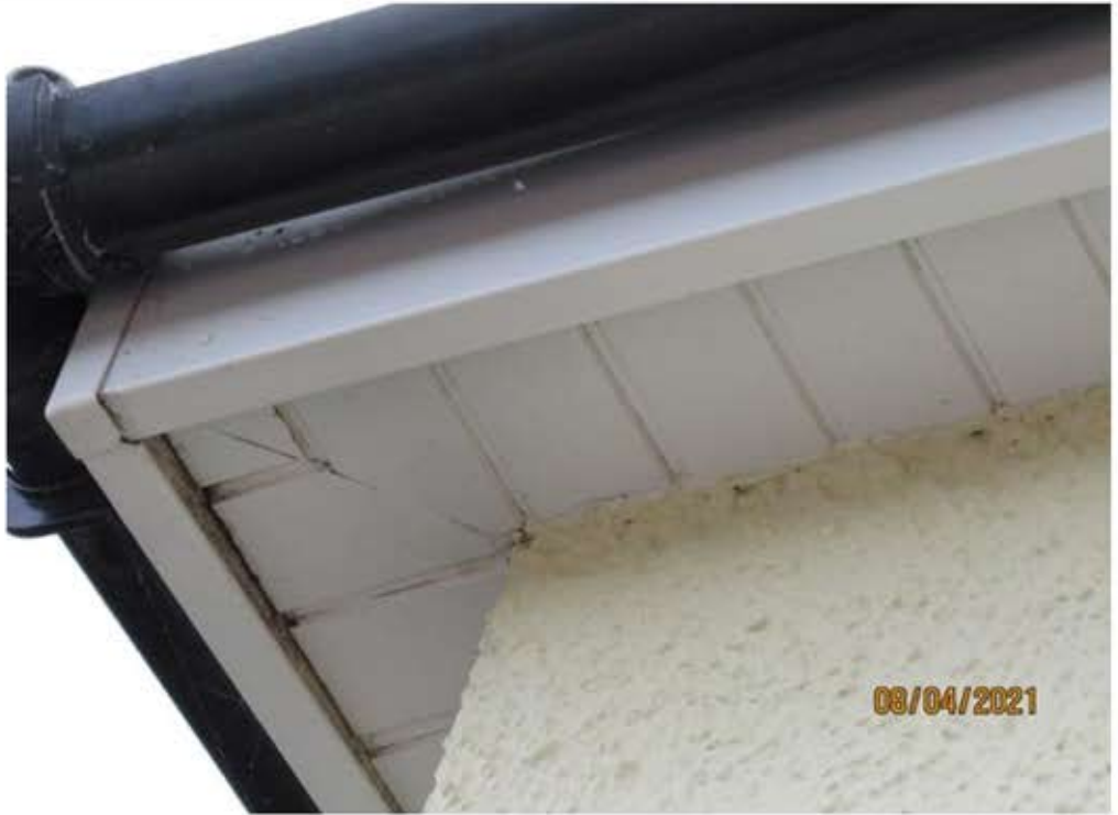
uPVC fascia and soffit boards but with no ventilation
