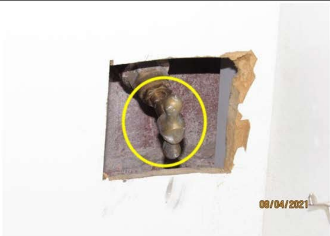
Internal water stop valve under kitchen sink
