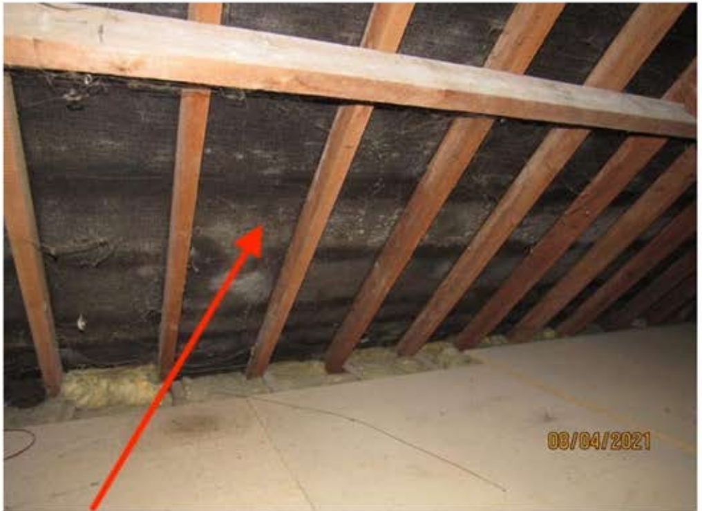
Water staining on underlay
