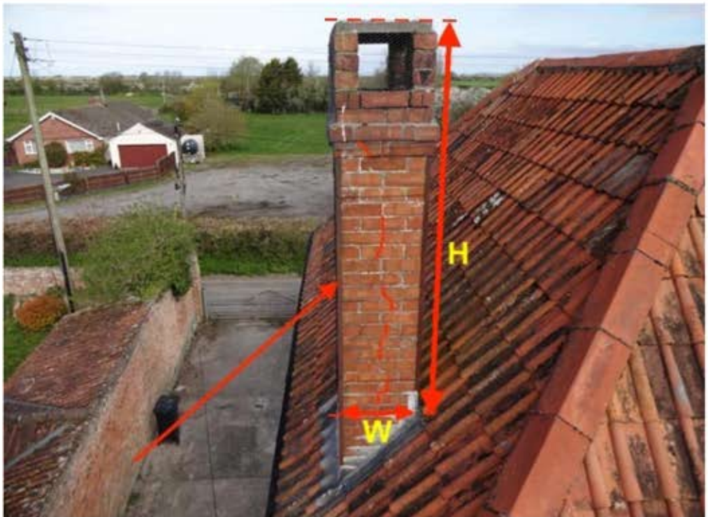
Vertical cracking in brickwork of west chimney stack, metal binders and slenderness ratio estimated at 4.35
