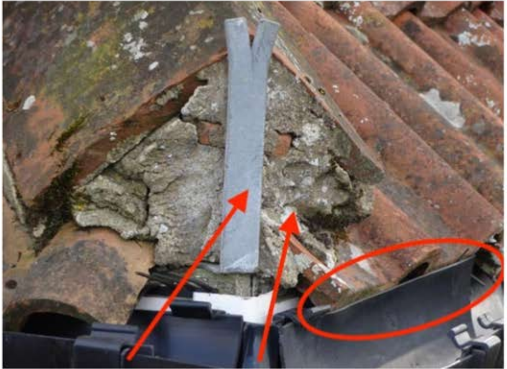
Poor workmanship at north-west corner
