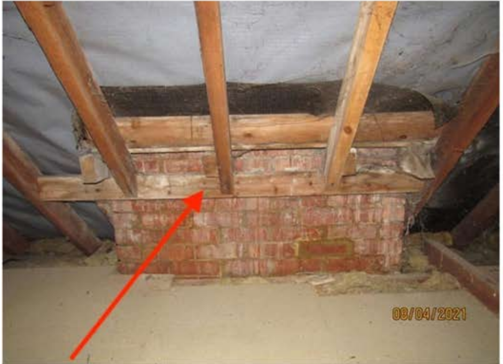
Water staining and high moisture meter readings in both chimney stacks
