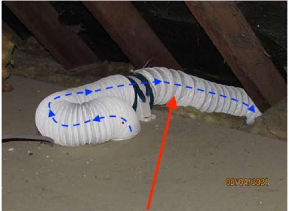
Flexible ventilation ducting from bathroom extractor fan to external vent grille in east soffit board
