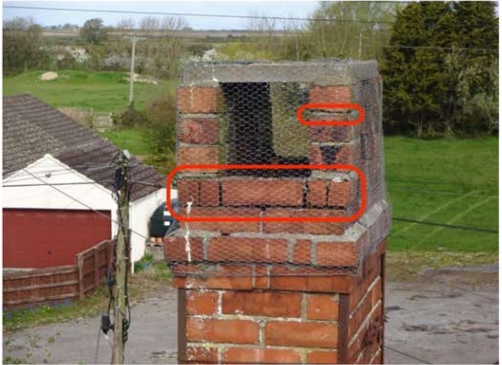
Missing mortar on west chimney stack
